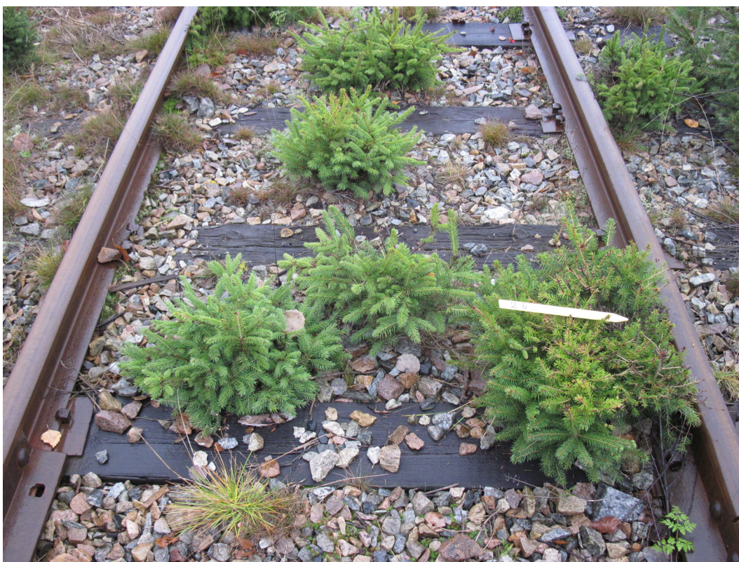
Figure 4. Weed level: 'Non-acceptable' Biomass value 26. Weeding measures using herbicides only is no longer possible. Mechanical weeding measures or cleansing of embankment must be carried out
