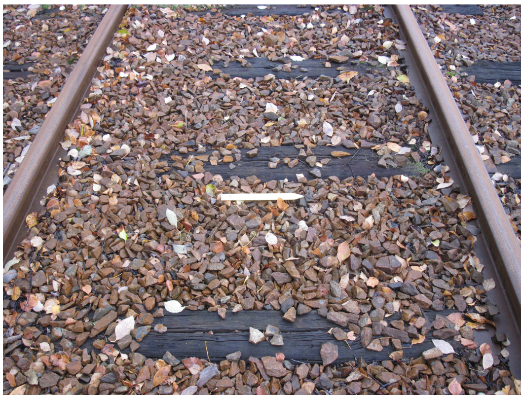
Figure 2. Weed level: ‘Non-existent’ Biomass value 1. An example of a railway line in proper condition.
